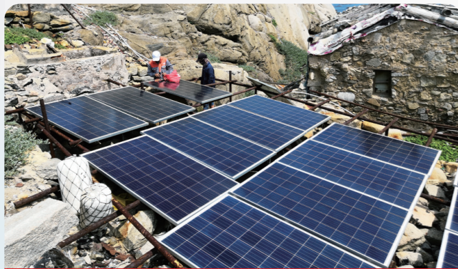
3KW PV Project in Nan'ao
