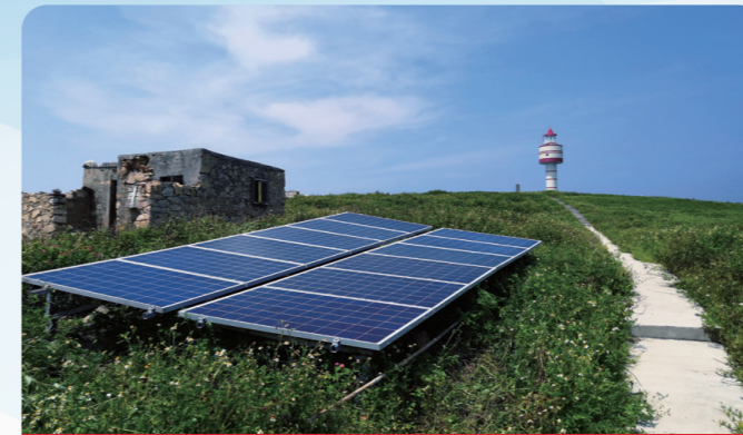
3KW PV Project in Nan'ao
