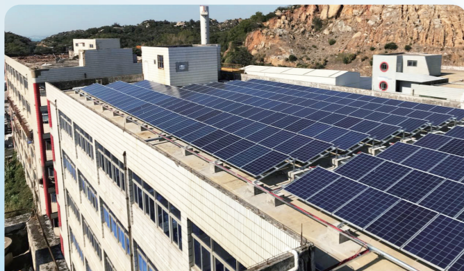
165KW PV Project in Guang'ao
