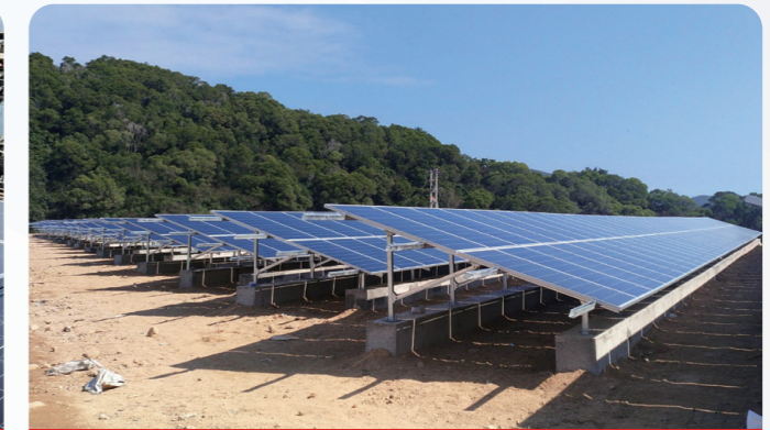
921.6KW PV Project in Nan'ao
