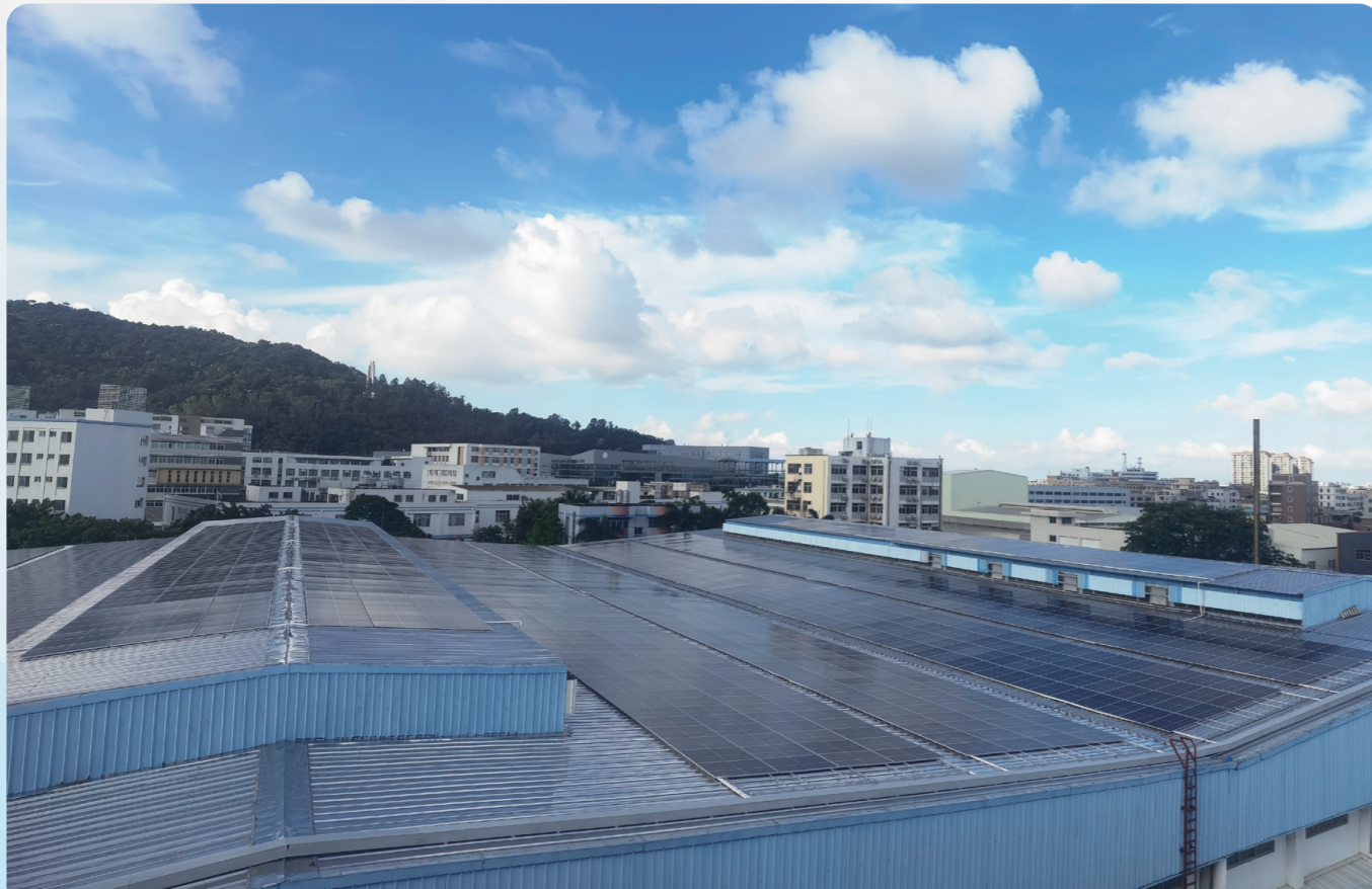
1.134MWp PV Project in Xiangfa
