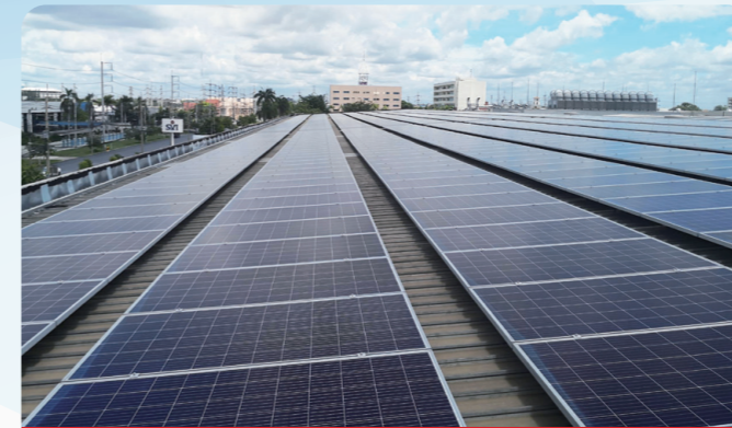
20MW Ground-mounted PV Station in the USA
