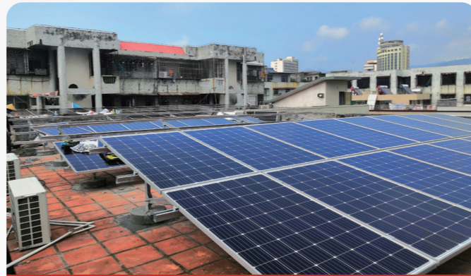
33.6kW Poverty Alleviation PV Project in Nan'ao
