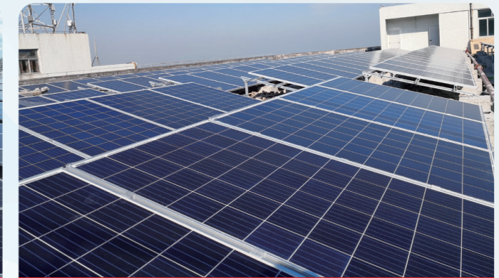
100KW PV Project in Donghu
